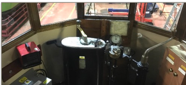
1017's new heater left hand side of photo
